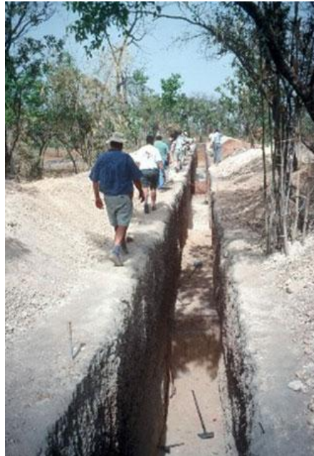
Figure 10: Large trenches such as this one in West Africa can be hazards to both wildlife and people unless reclaimed. © lamgold.
