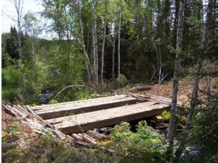
Figure 17: A well-constructed bridge can minimize stream disturbance, carry heavy equipment and need not have high cost. © Golden Band.
