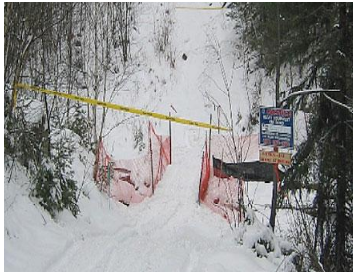
Figure 20: Winter stream crossing. Note use of snow fencing for guidance, warning signs and silt fencing. © Noranda/Falconbridge
