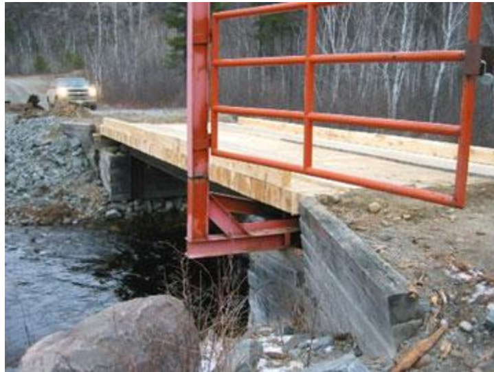
Figure 18: Good example of a steel girder bridge with wooden deck and stone-filled cribs. Locking gate can be used in this case to control access.© Noranda/Falconbridge
