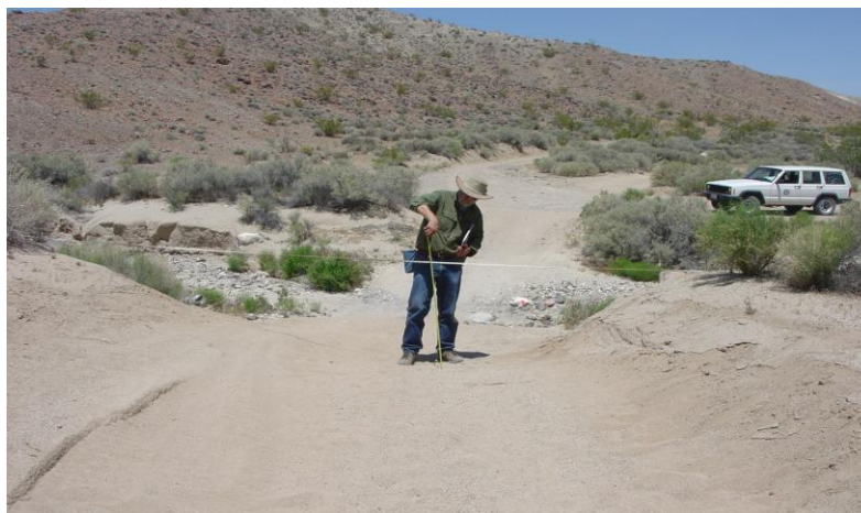
Figure 29: Photograph demonstrates depth of erosion due to cut and soil loss on off road vehicle trail. Tape has been strung horizontally to depict the unaffected ground surface. Last Chance Canyon, California (picture courtesy of San Diego Office, California State Parks)
