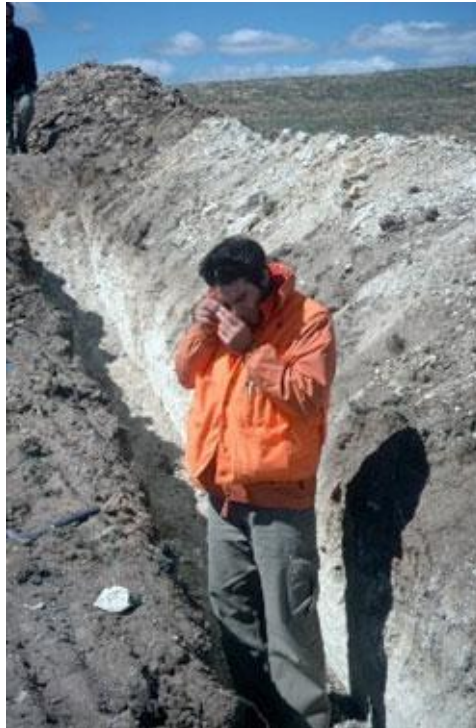
Figure 11: Trenching can leave a major scar on the landscape unless reclaimed. The muck pile from this trench in Argentina will be used as backfill upon completion of work. © Iamgold.
