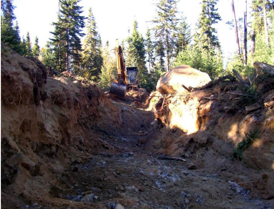
Figure 21.7: Trenches should have one end with a gentle slope for easy exit. © Lorne Burden
