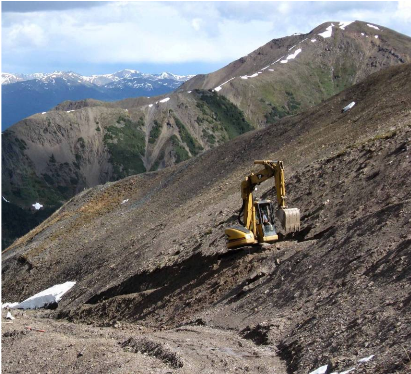
Figure 21.1: Do not stand or work downhill from heavy equipment in case it rolls or knock debris downhill © Matt Turner
