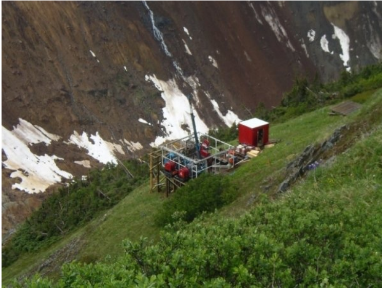
Figure 20.1: Drilling on steep slopes requires attention to drill pad stability and fall prevention. © Hy-Tech Drilling Ltd.
