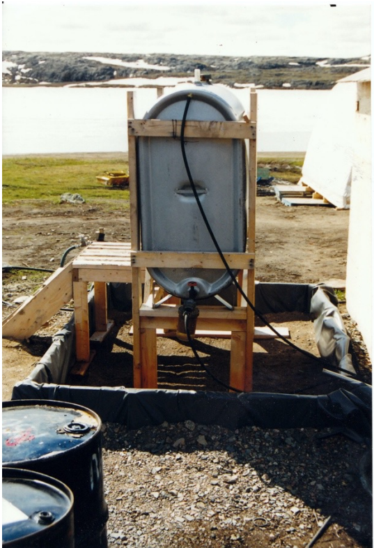
Figure 18.7: A refillable heating oil tank and berm lined with chemical resistant fabric. © Bill Mitchell
