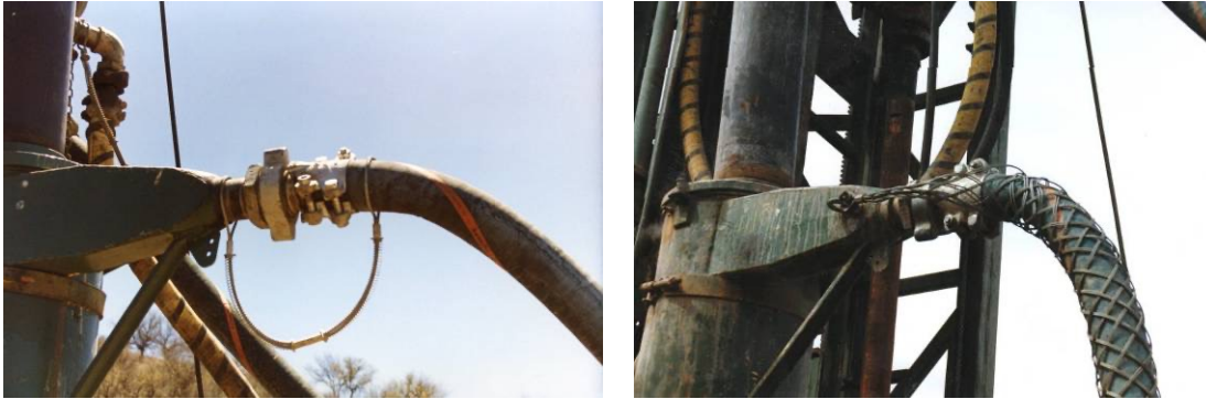
Figure 20.5: Standard whip check (left) and cable stocking whip check (right) © Bill Mitchell
