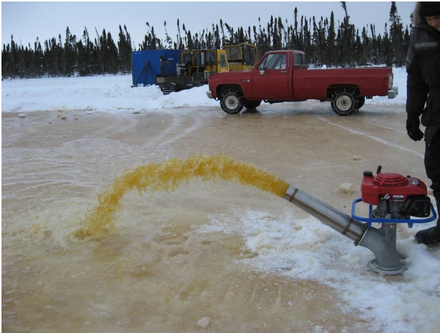
Figure 20.2: Building a thicker drill pad by flooding the ice to create lifts that freeze in 12-24 hours. © Chris Pedersen
