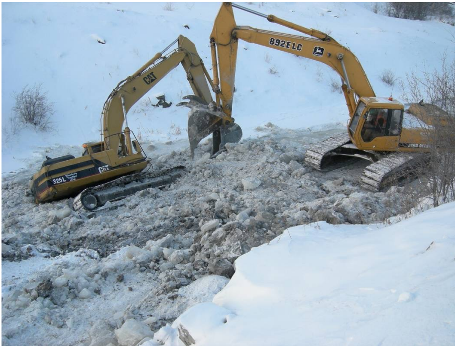
Figure 21.5: Measure the thickness before using heavy equipment on ice, especially on frozen rivers and streams where ice thickness is always variable. © Steve Millar
