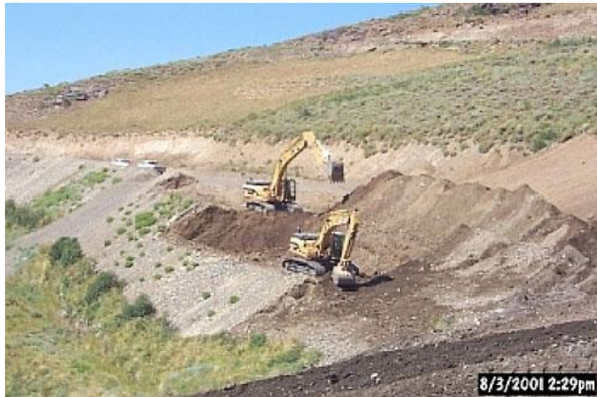
Figure 68: Road reclamation usually involves two excavators working in tandem. The original slope is restored by cutting down the upper slope and pulling up material from the lower slope. © AngloGold.
